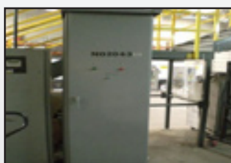
600 AMP ATS ASCO $1,950 Ser #FP87387 480v, 4p, 3r, Forklift skids. (N02043)
